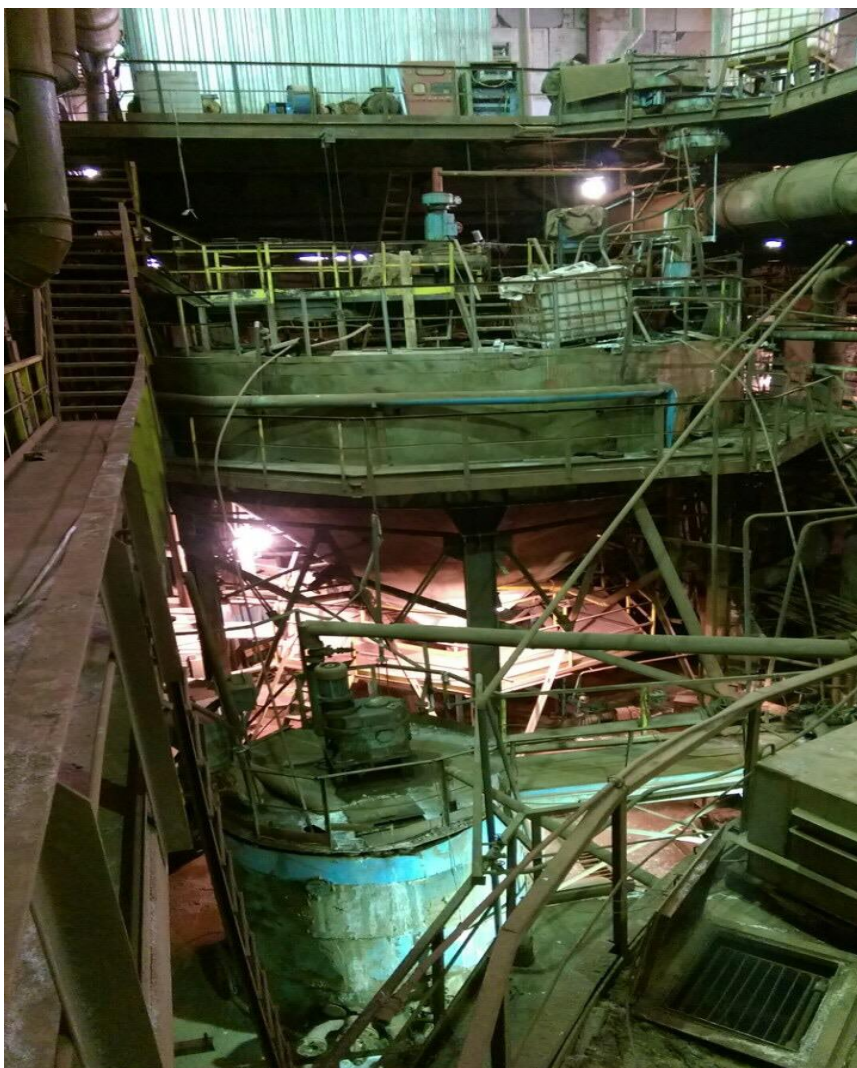
Fig. 1. A part of the experimental-industrial plant of the red mud processing unit.
